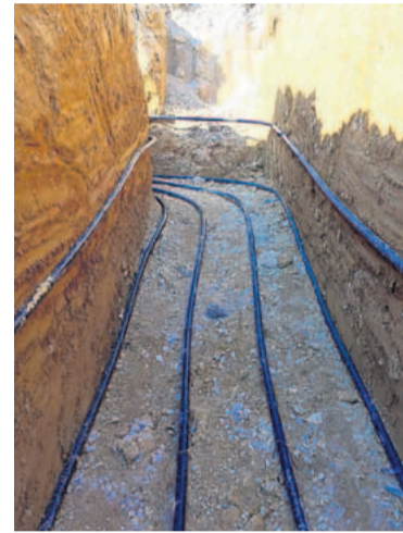
This photo taken early on in the project shows the excavation required to bury the geothermal at least 6 feet down, where the temperature of the earth is a near constant 55 degrees.
