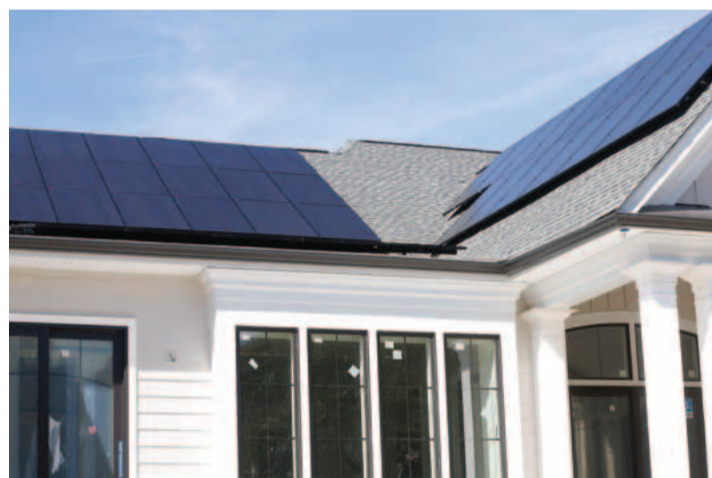
Advanced photo-voltaic solar panels are installed on the the south-facing roof, out of sight from the front of the house.
