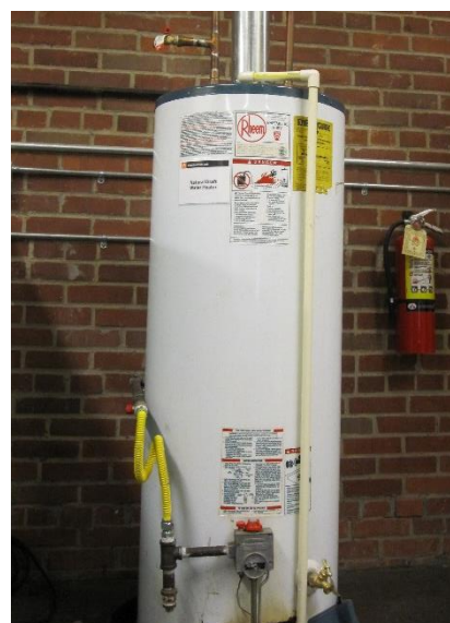
Gas Storage Tank
