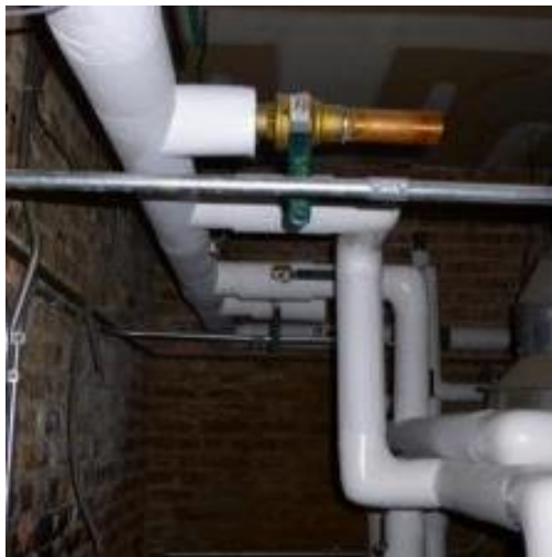
Insulate 100% of hot water pipe
