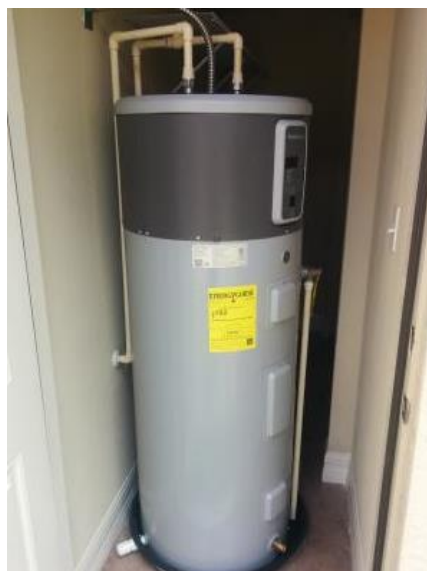
Electric Storage Tank
