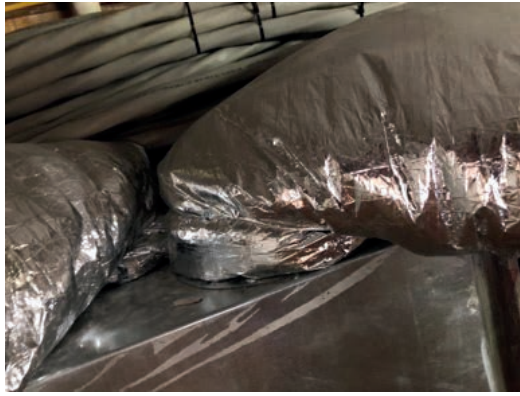
Figure 6: Unsealed and poorly supported duct takeoff
