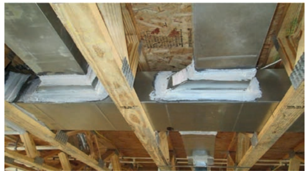
Figure 4: Well sealed supply-to-trunk connection
