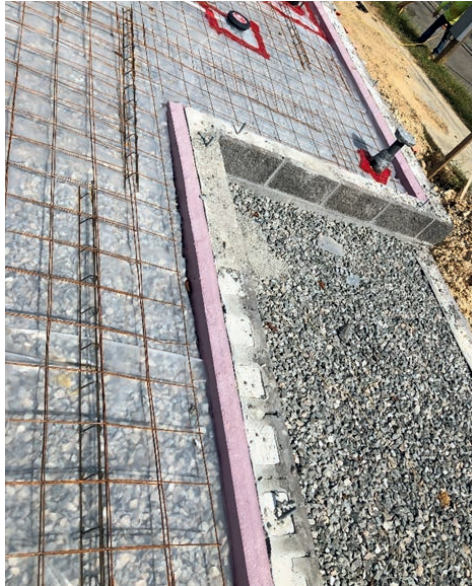
Figure 4: Stem Wall insulated to height of Slab. Insulation to be cut at 45 degree angle away from wall (Code Section R402.2.10)
