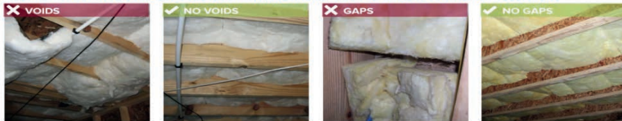
Figure 2: Various examples of good and bad installations
