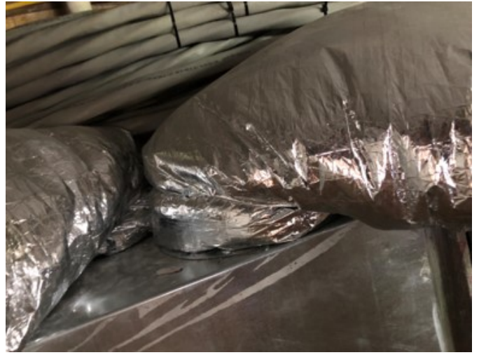
Figure 6: Unsealed and poorly supported duct takeoff
