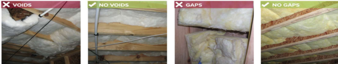
Figure 2: Various examples of good and bad installations
