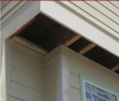
✗ NO RIGID AIR BARRIER
