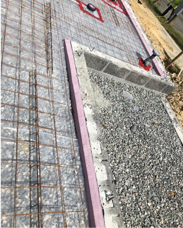
Figure 4: Stem Wall insulated to height of Slab. Insulation to be cut at 45 degree angle away from wall (2018 VRC Code Section N1102.2.10 (R402.2.10))
