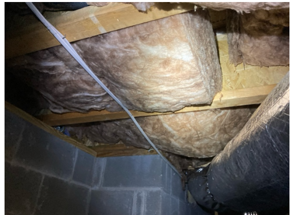
Figure 2: Traditional wire stays compress batts, support irregularly, and fall out - Insulated floor over vented crawl in 8-month-old Virginia home. Photo: Viridiant
