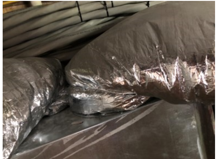
Figure 6: Unsealed and poorly supported duct takeoff. The immediate 90 degree turn should use hard duct.
