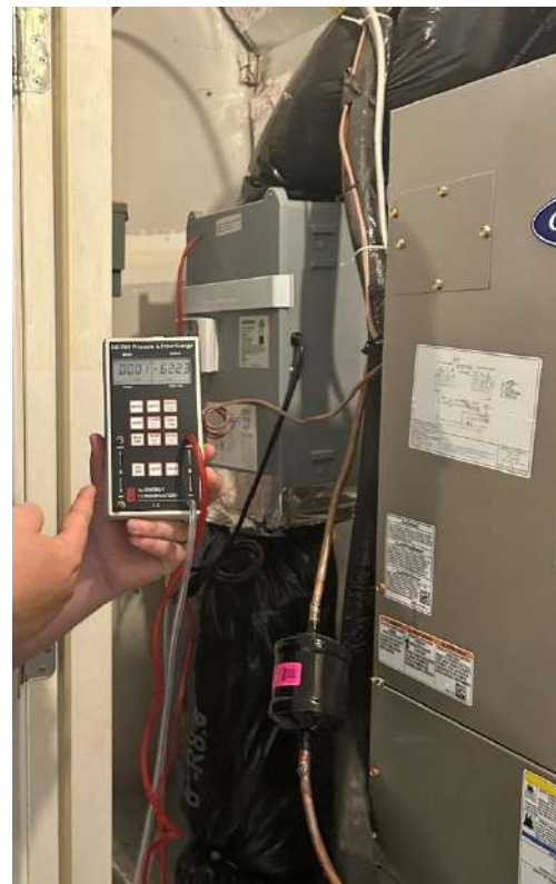
Figure 3: Image: Measuring whole-home ventilation air flow via probes in the energy recovery ventilator.
